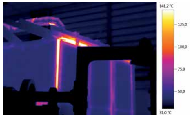
Industrial kiln with faulty insulation.
